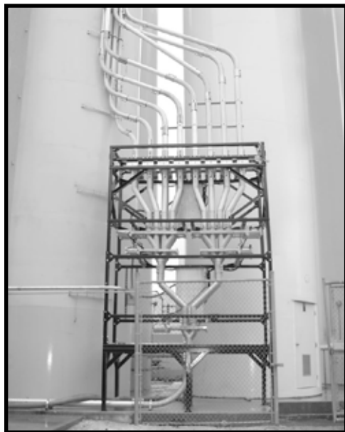
Vortex Wye Line diverters conveying plastic pellets from two rail cars to eight silos.
