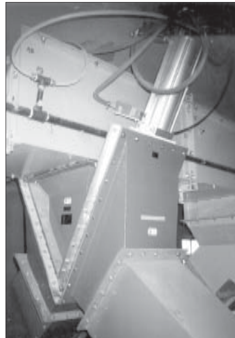
GRAVITY VEE diverter mounted beneath a drag conveyor at the grain elevator serving ADM Milling Co.’s Carthage, MO, flour mill can divert incoming wheat into one of two storage tanks or to both simultaneously. Photo courtesy of ADM Milling Co.
